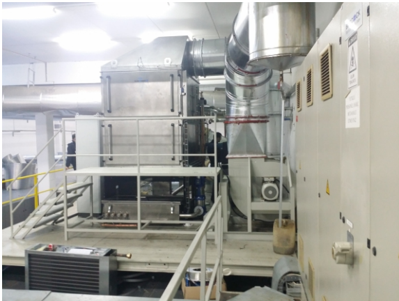
The KMA ULTRAVENT was installed above the stenter.
